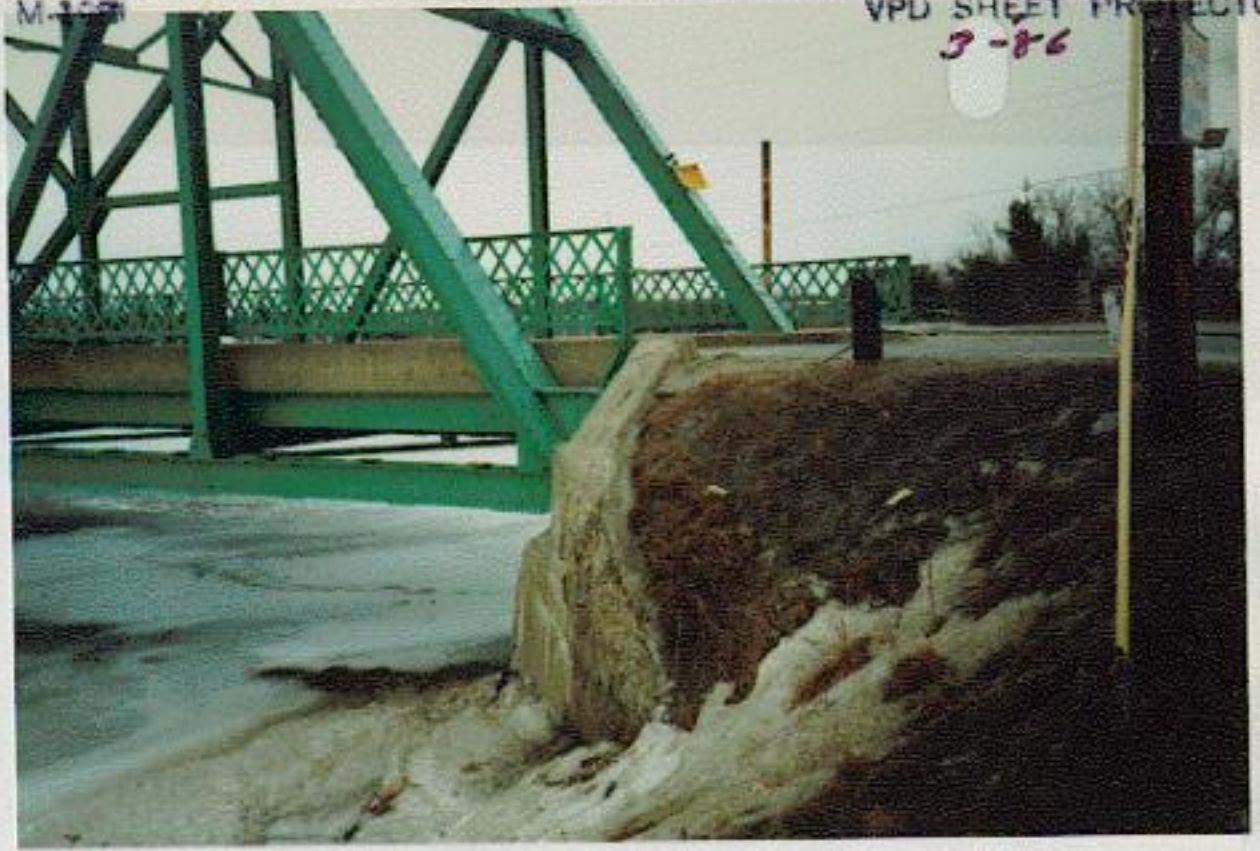
Heavy wingwall sealing
