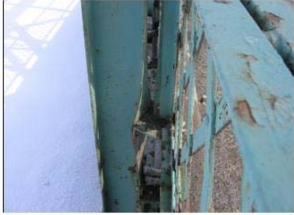
Damaged truss post/connection
