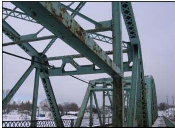
Truss - note paint failure
