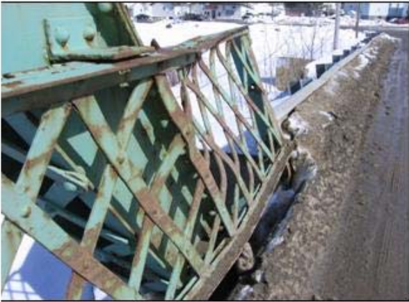
Bridge rail damage
