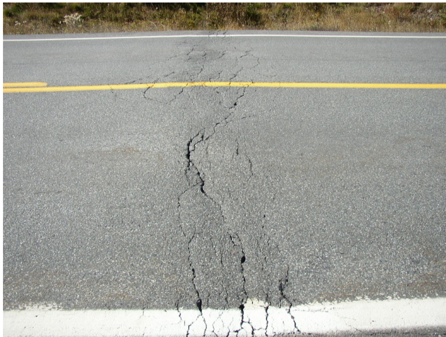
Photo 5: Cross Pipe 4 Transverse Cracking
