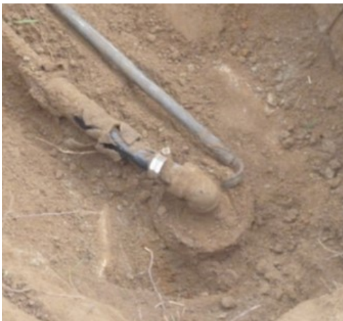
Figure 4. Buried well. Photo courtesy of Lakeland Water Pump Co.
