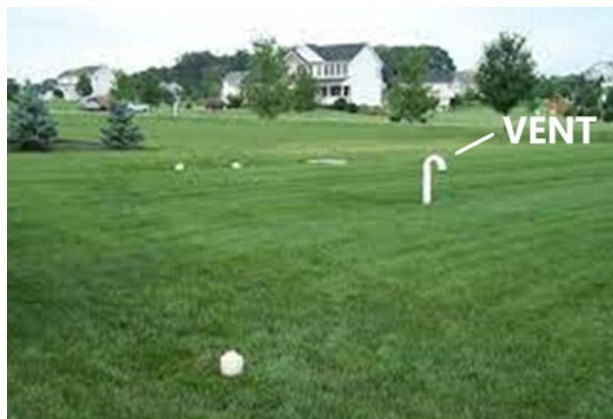
Figure 8. Ventilation pipes are sometimes specified in the septic system design. When they are used, the plumbing vent in the home roof acts as the high-end vent and the vent at the end of the system acts as the low-end vent. Vents often resemble “candy canes” without the stripe, but they can be disguised as birdhouse poles. In many cases, vents in home systems are not used.. Photo courtesy of thedrainbrain.com.
