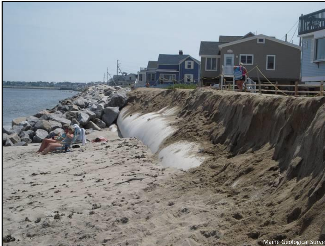
Figure 6. Undermining of the geotube remains a problem due to the combined effects of storm events and increased ("end effect") erosion at the northern end of the seawall.
