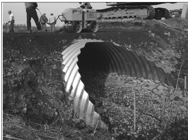
This culvert seems large enough to allow a stream channel to form in the bottom.
