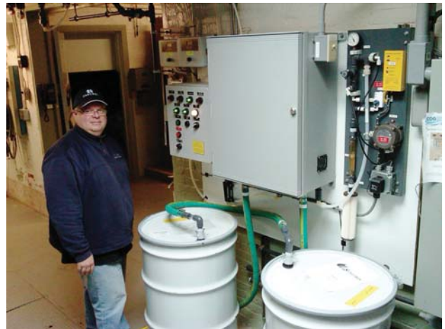
Bill Snyder, Treatment Plant Manager, stands next to KKW's new chlorine dioxide treatment system. Photo courtesy of KKW.
