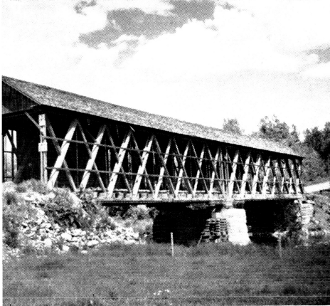
WATSON'S SETTLEMENT BRIDGE in Littleton with side boards removed showing "bones" of a typical covered bridge. Howes truss used iron rod uprights. Bridge was "tuned up" periodically by tightening bolts.
