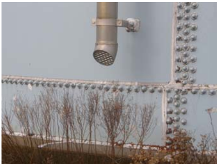
Tank overflow with screening to prevent entry from animals
