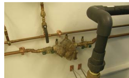
A testable backflow prevention device on a treatment feed line
