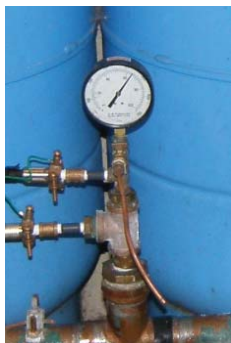
A minimum of 20 psi should be maintained at all times and under all conditions throughout water system
