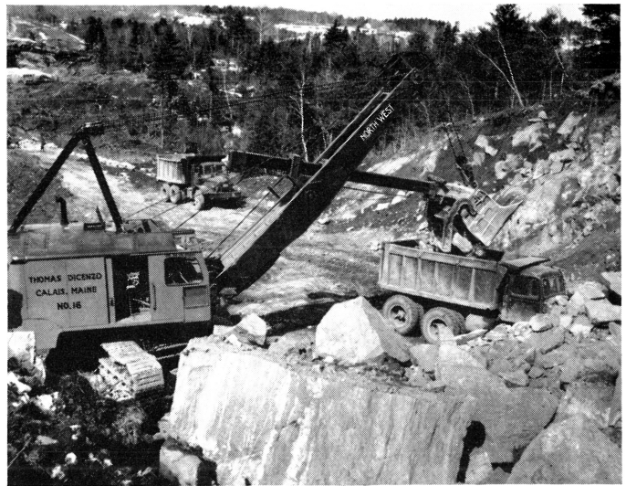
THE BIG BITE of a 2½ yard shovel makes quick work of loading rock blasted from a head of ledge. 60,000 yards of ledge will have to be moved in building this 2.2 mile section of U. S. Route 1.
