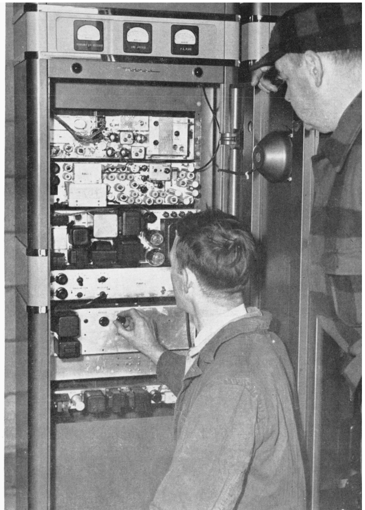
ROBERT PARKER, Radio Supervisor and Alvin Allen, Technician, check over a repeater transmitter which is located in a cement block building at a mountain top location. The transmitters are checked at regular intervals as insurance against breakdown. Most of these stations have automatic electric generators which go into action immediately on power failure, thus adding additional insurance against being off the air.
