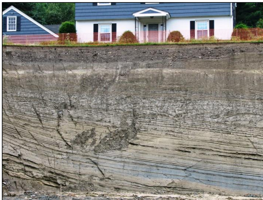
Figure 3.17. Clay-silt beds of the Presumpscot Formation, exposed at a 2008 construction site on the east side of the Kennebec River valley in Augusta.
