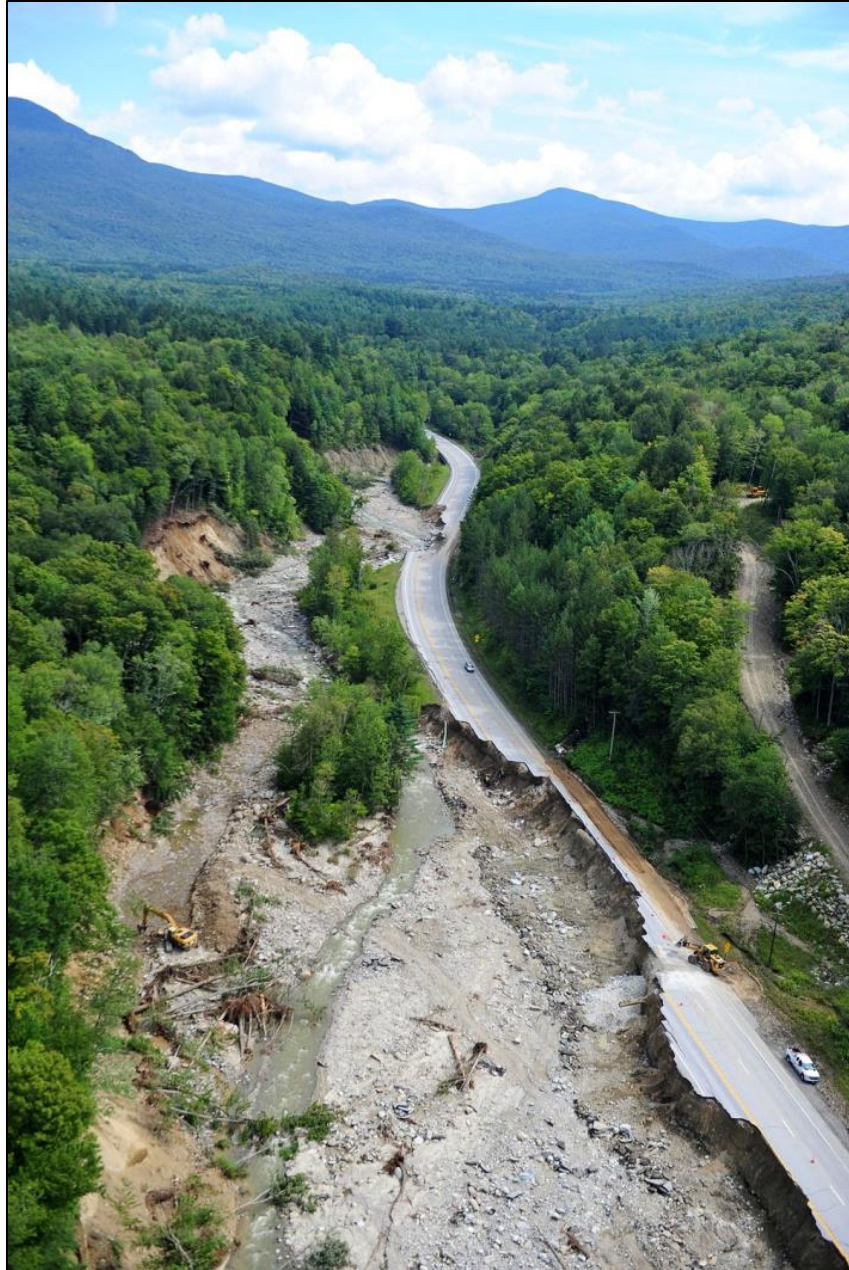
Figure 5.3. Severe erosion along U. S. Route 4, Mendon, Vermont, resulting from tropical storm Irene in 2011. Photo by Lars Gange & Mansfield Heliflight.
