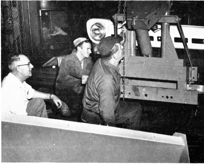
Voyle Reed (left) checks the installation of a front mount on a Ford F 600, one of the 150 private plows used throughout the State. Twenty-six new R-20 Ross blade plows were purchased this year, most of which will be used on hired trucks. Mechanics are Donald Drake and Judson Stinson.
