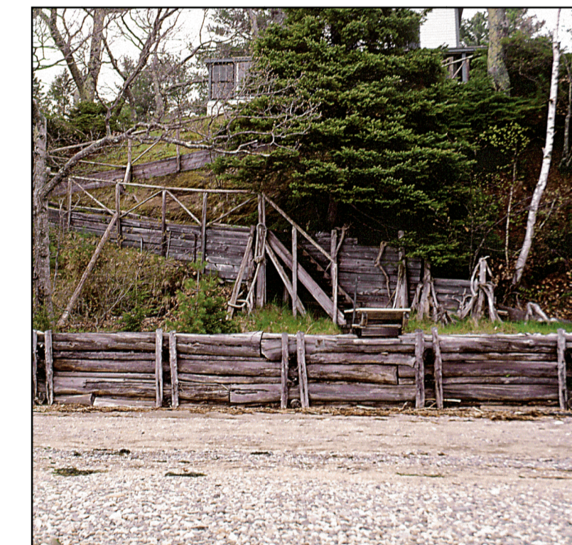
Stable bluff with a vegetated bluff face and an armored shoreline. The bluff face is fully vegetated and supports a mature stand of vertical trunks. The presence of a wooden bulkhead suggests that erosion has occurred in the past.
