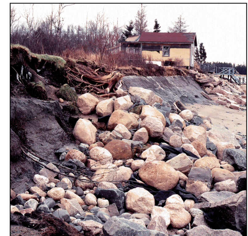
Highly unstable bluff with an unvegetated bluff face and an armored shoreline. This armored bluff is eroding despite an effort to shore it up with riprap, or loosely piled stone blocks. Maintenance at this site could improve bluff stability.
