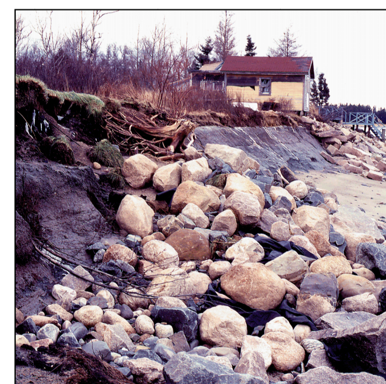
Highly unstable bluff with an unvegetated bluff face and an armored shoreline. This armored bluff is eroding despite an effort to shore it up with riprap, or loosely piled stone blocks. Maintenance at this site could improve bluff stability.
